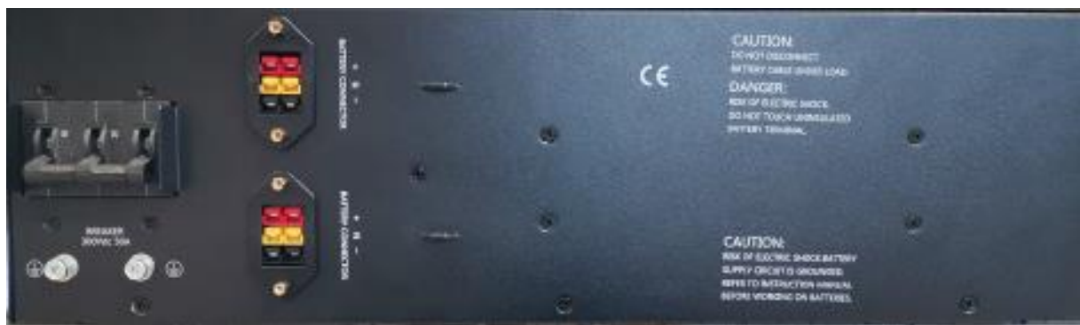
BATTERY CABINET REAR VIEW
